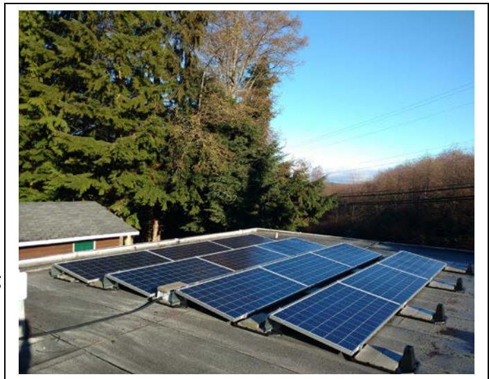
RDMW Office Solar/Battery back-up power system
