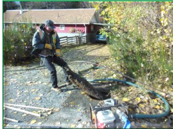
Figure 7 Woss Sewer Plug 2013
