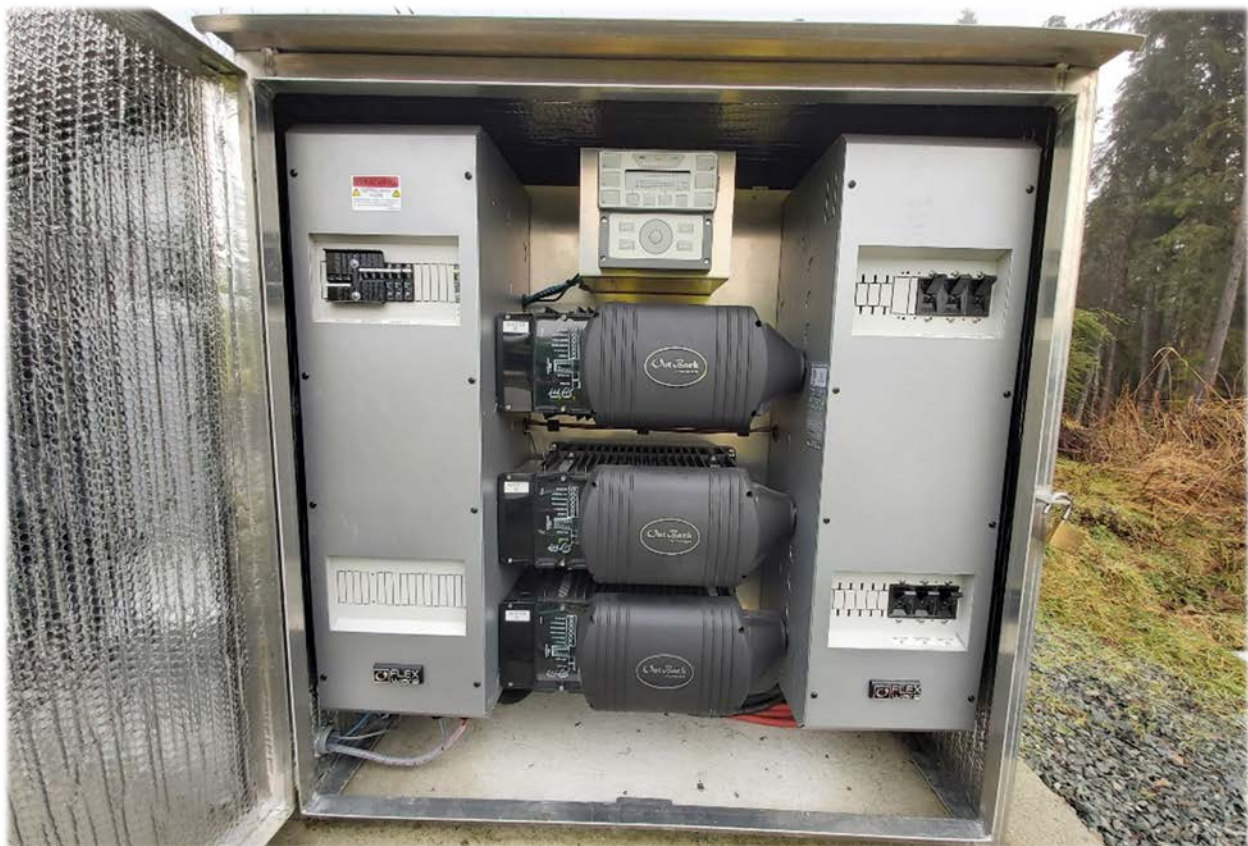
Coal Harbour Wastewater Power System
