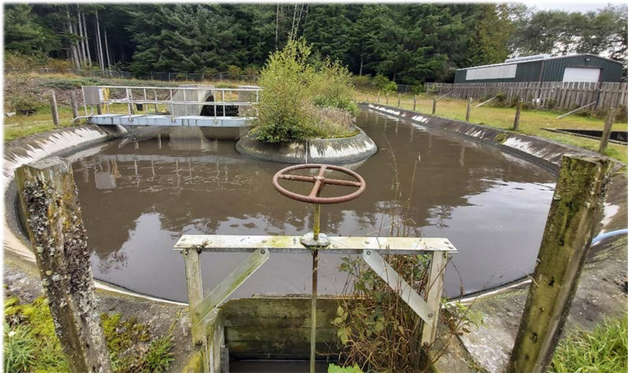
Sointula Wastewater Treatment Plant
