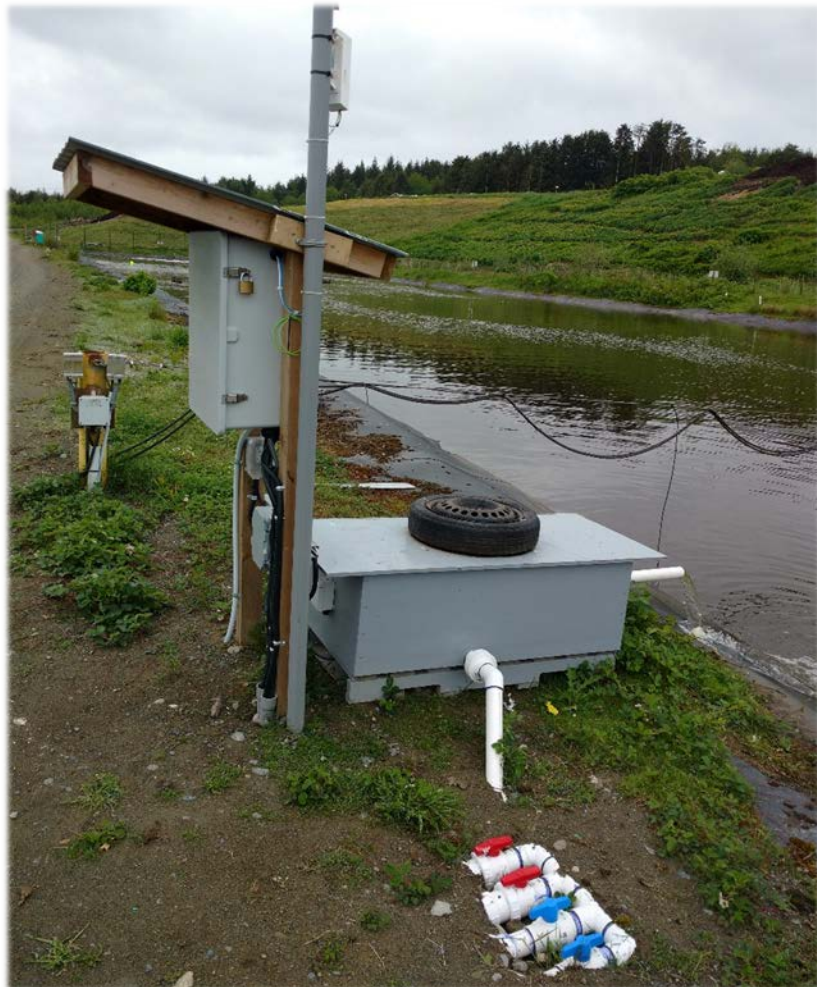
Leachate Monitoring System:
