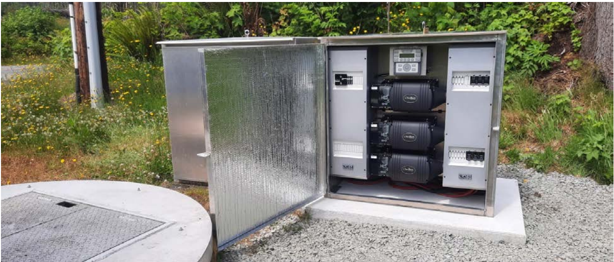
Figure 2: Coal Harbour Lift Station 2 Invertors
