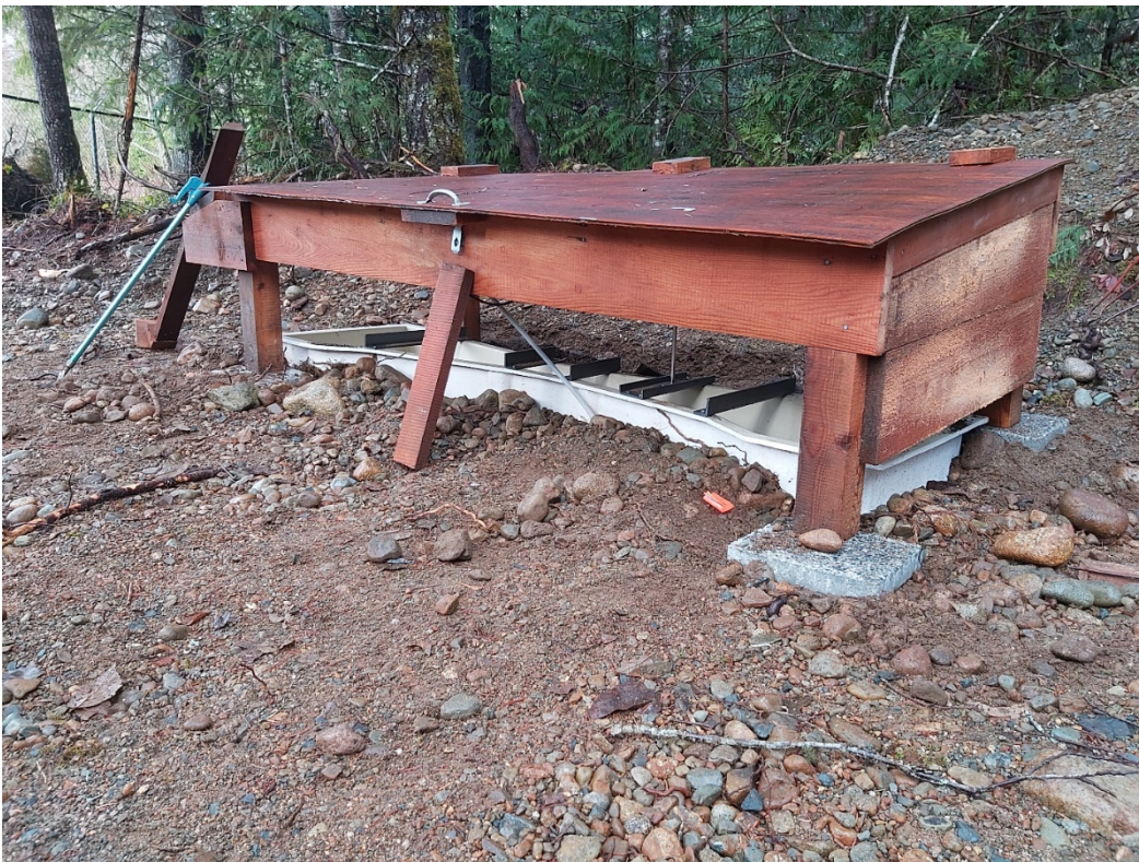
Figure 2: Flume complete with cover and sensor
