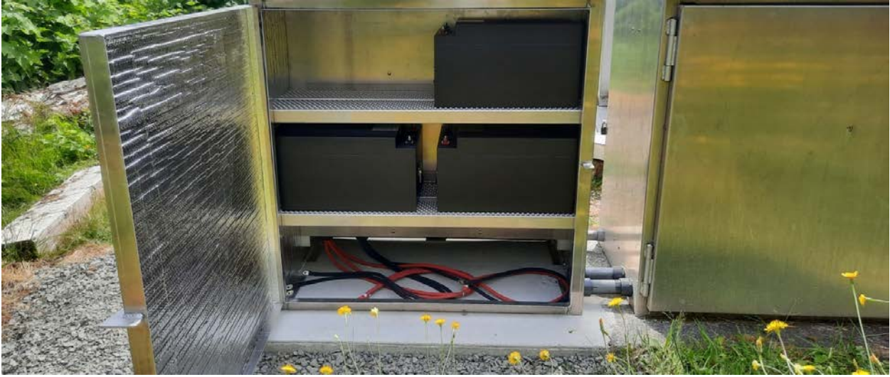
Figure 1: Coal Harbour Lift Station 2 Lithium Batteries
