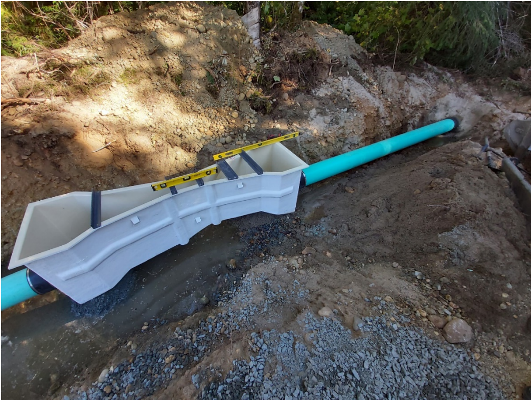
Figure 1: 6" Parshall flume installation with new 10" SDR pipe and couplers
